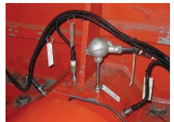
A typical example of the mounting of sensors onto a machine
